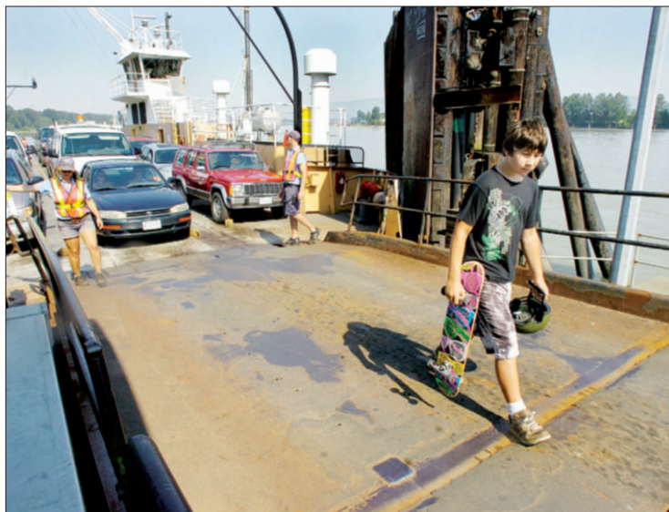
The aging Albion Ferry dock, which back in its day saw thousands a day driving over it as they loaded and unloaded off the ferry, now needs to be removed, according to Kwantlen First Nation. They are paying security to prevent more problems.
